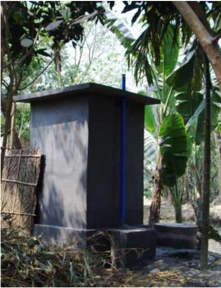
Well-built latrine with ventilation pipe and off-set pit (Bogra District, Emdadul Hoque photo, 2010)
